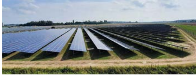
13.00 MWp Type: Ground Mounted Year: 2019 Location: The Netherlands Status: Completed
