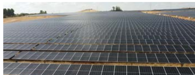
20.00 MWp Type: Ground Mounted Year: 2021 Location: Spain Status: Completed
