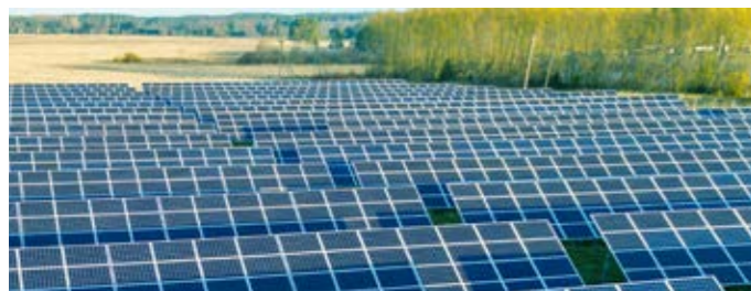
9.40 MWp Type: Ground Mounted Year: 2018 Location: Turkey Status: Completed
