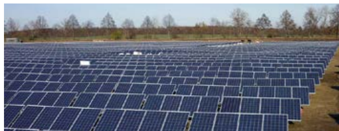
3.40 MWp Type: Ground Mounted Year: 2018 Location: Turkey Status: Completed
