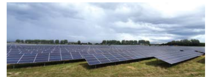
14.00 MWp Type: Ground Mounted Year: 2019 Location: The Netherlands Status: Completed
