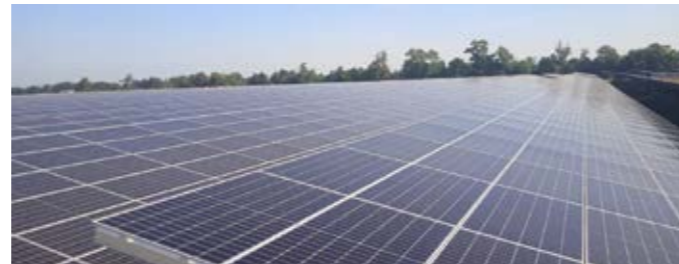
28.00 MWp Type: Ground Mounted Year: 2021 Location: The Netherlands Status: Completed
