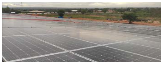
2.20 MWp Type: Rooftop Location: Mozambique Year: 2020 Status: Completed
