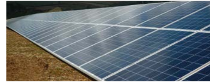
64.00 MWp Type: Ground Mounted Year: 2020 Location: The Netherlands Status: Completed
