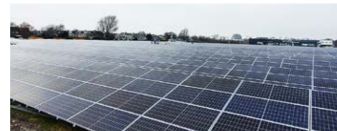
3.10 MWp Type: Ground Mounted Year: 2020 Location: The Netherlands Status: Completed
