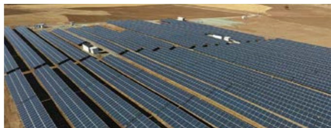
11.00 MWp Type: Ground Mounted Year: 2017 Location: Turkey Status: Completed
