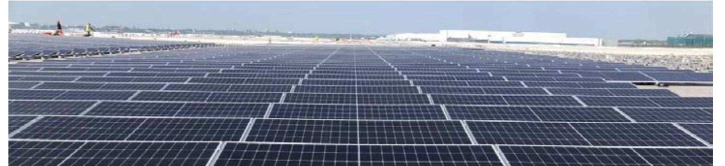
2.55 MWp Type: Rooftop Year: 2021 Location: The Netherlands Status: Completed
