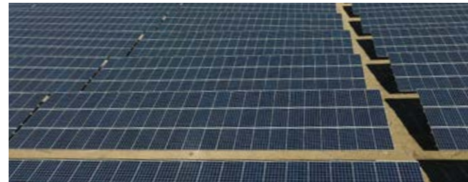
5.80 MWp Type: Ground Mounted Year: 2020 Location: The Netherlands Status: Completed
