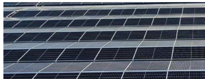
1.25 MWp Type: Rooftop Location: Germany Year: 2019 Status: Completed
